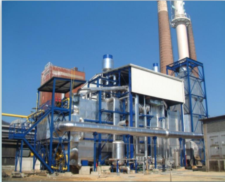
silencers installed on the roof with optimum noise and safety performance
