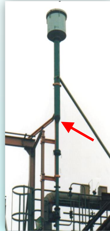
no insulation small blow off pipe
