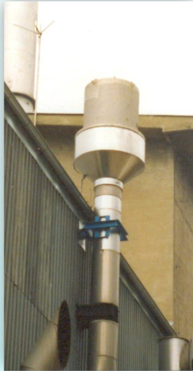
insulated blow off pipe
