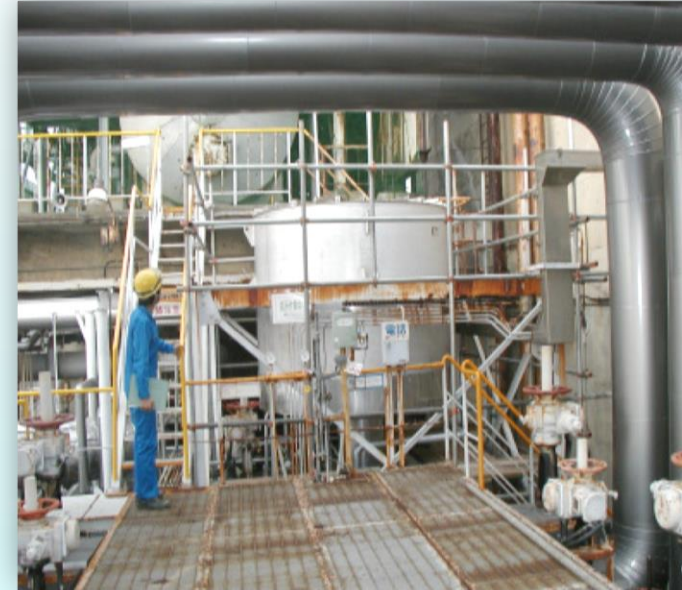
installation inside a building
